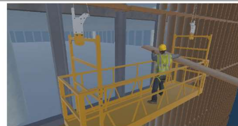
Figure 20 Long protruding vertical fins that need to be installed manually by workers on a gondola
